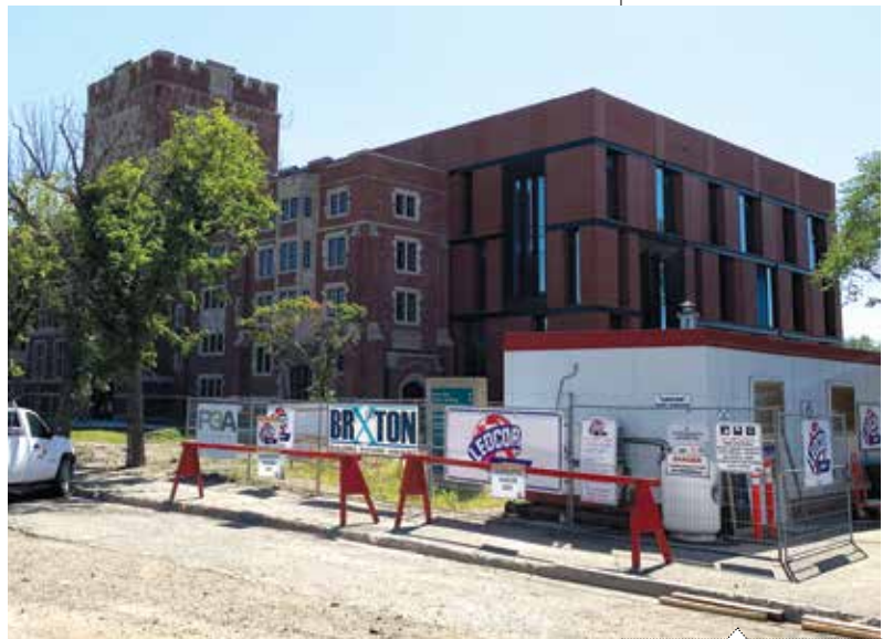
The $60M College Avenue Campus Renewal will maintain the legacy of the University of Regina’s historic campus located on the edge of downtown Regina.
